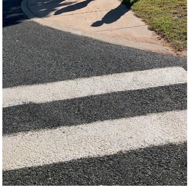
Vision Boulevard, south side, ramp at high school – needs to be made ADA-compliant
