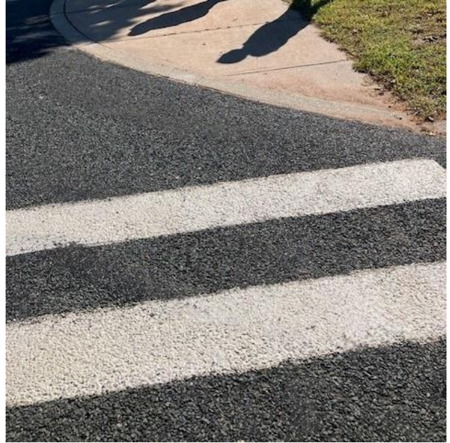
Vision Boulevard, south side, ramp at high school – needs to be made ADA-compliant
